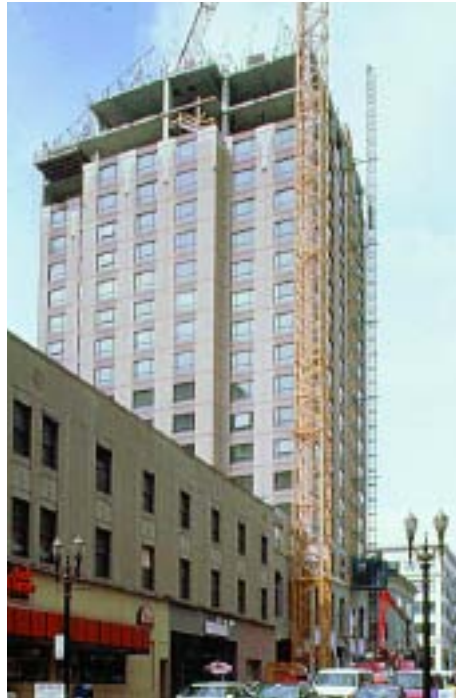
The new 20-story Westin Hotel in Portland, Oregon, met construction deadlines using desiccant drying.
