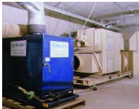
Munters desiccant dehumidifiers located in the basement, pumped dry air to the floors above.
