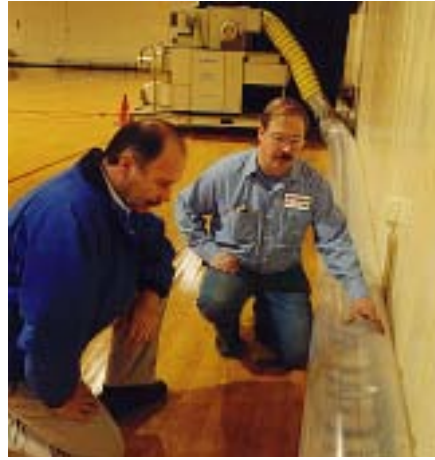
Jim Ammann inspects Munters gym floor drying configuration, which pumped dry air under the wet floor.
