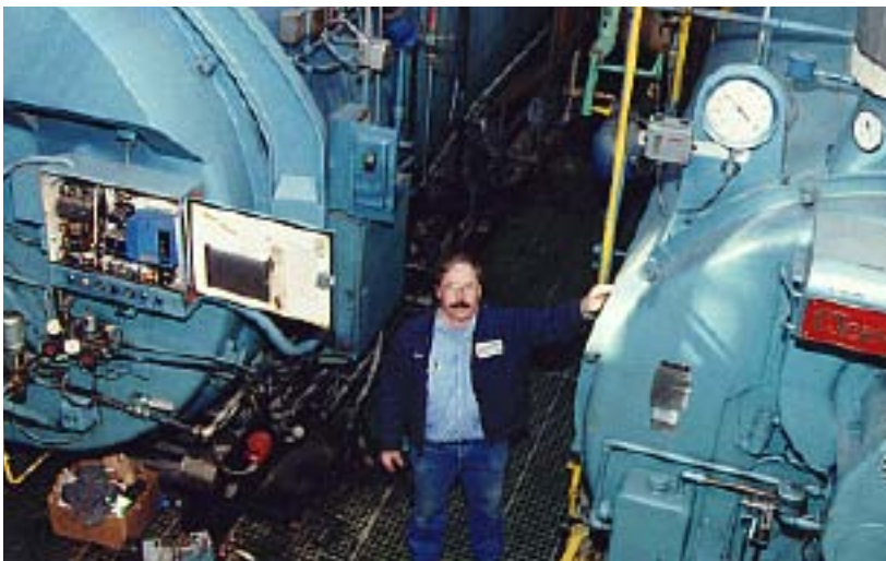
Jim Ammann points to the high-water mark in Wentworth's boiler room. Munters dried the boiler room, protecting the equipment. "We didn't even have to repaint it," said Ammann.
