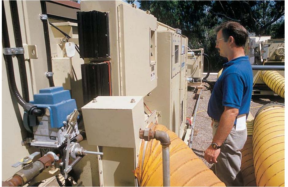
Munters' temporary humidity/temperature control system was built up from equipment hoisted on to the Museum roof with a crane. It kept an area nearly 400,000 cubic feet at 72° F and 55% RH.
