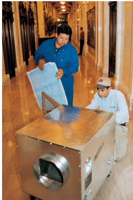
Munters technicians change the HEPA filter in an air scrubber. Air scrubbers were used to remove fine dust particles from building air.
