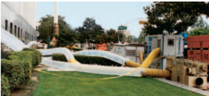
Munters was the only company that could start drying with the power to the courthouse shut off. Self-powered units were on site and drying before the basement was pumped.
