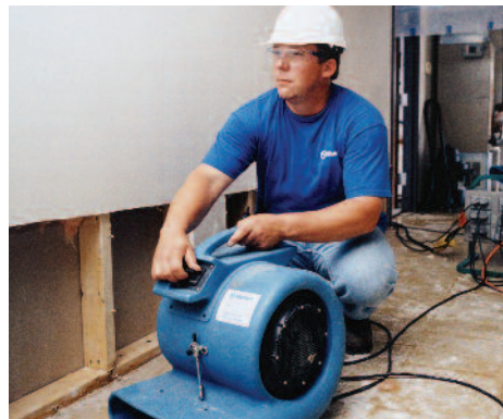
Left, Munters provides controlled demolition, removing unsalvageable drywall, allowing dry air to reach into wall cavities. Soot, smoke damage and odors are treated, preparing the building to be safely re-occupied.
