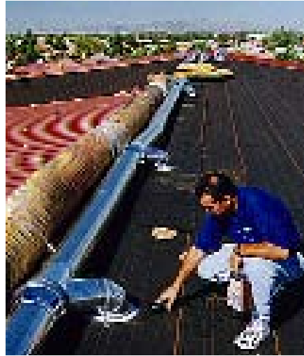
A plenum running along the peak of the roof conducted dry air from the dehumidifiers into the roof structure. The air flowed down to the eaves, where Munters measured its humidity level to monitor the drying process.
