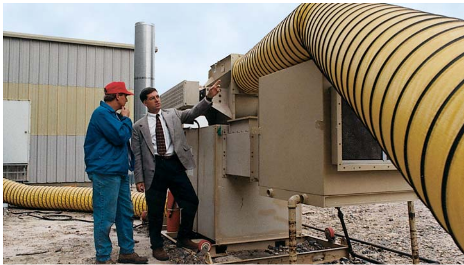
Munters MCS rental dehumidifiers controlled humidity for four months.
